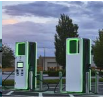
EV Charging Station 充電站
