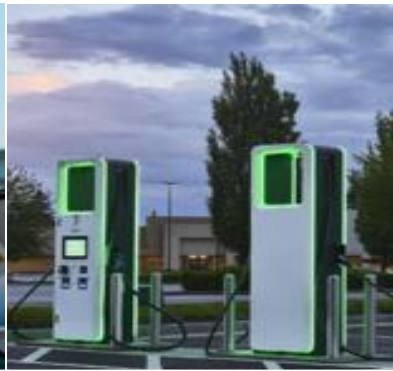
EV Charging Station 充電站
